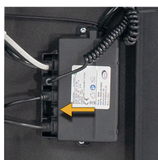
BEFORE: CONTROL BOX WITH THE CAP
