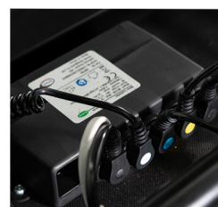
CONTROL BOX CONNECTED WITHOUT THE CAP
